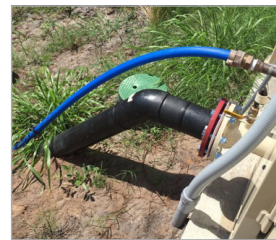
Incoming suction line and self-cleaning screen flush nozzle return line.
